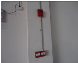
Photo of fire safety equipment Fire alarm.JPG
