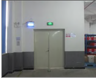
Photo of fire safety equipment Safety exit with emergency light and exit sign.JPG
