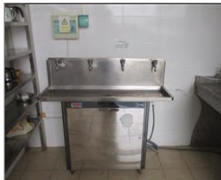
Photo of the sanitary facilities Potable water.JPG
