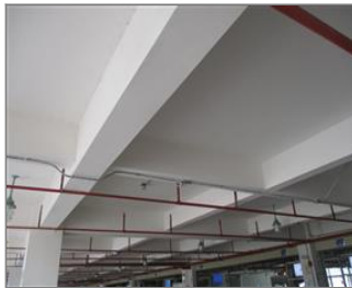
Photo of fire safety equipment Sprinkler system.JPG
